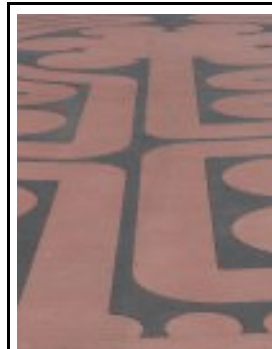
Our polymer concrete labyrinth at Our Lady of Victory Hospital in Stanley, Wisconsin, still beautiful two years after installation.
